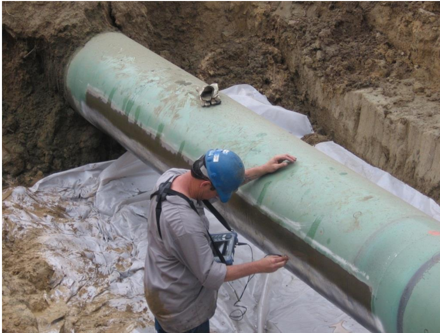
Field Ultrasonic Testing of Identified Pipe Joint's Long Seam for Potential Weld Imperfections "Penetrators"
